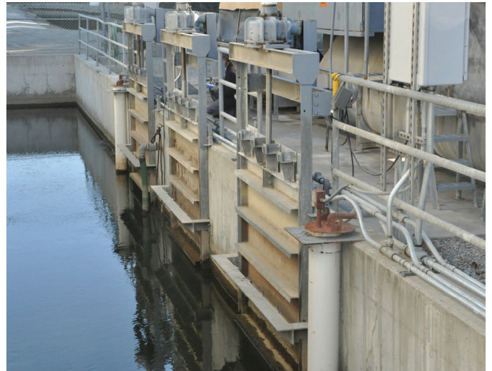
72-inch gates at UWCD's Moss Screen facility
