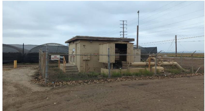
Photograph 4. View of the existing PVCWD-operated Well No. 7 at the proposed pump station site, facing northeast.
