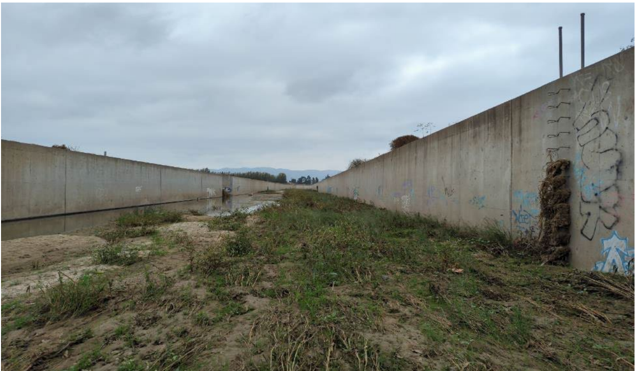
Photograph 22. View of Revolon Slough as it travels south and outside the Study Area. Note drift deposits along the left (west) bank (Aspect: southeast; September 13, 2023).
