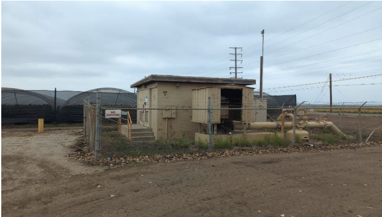
Photograph 7. View of the existing PVCWD-operated Well No. 7 in the eastern portion of the Study Area (Aspect: northeast; September 13, 2023).
