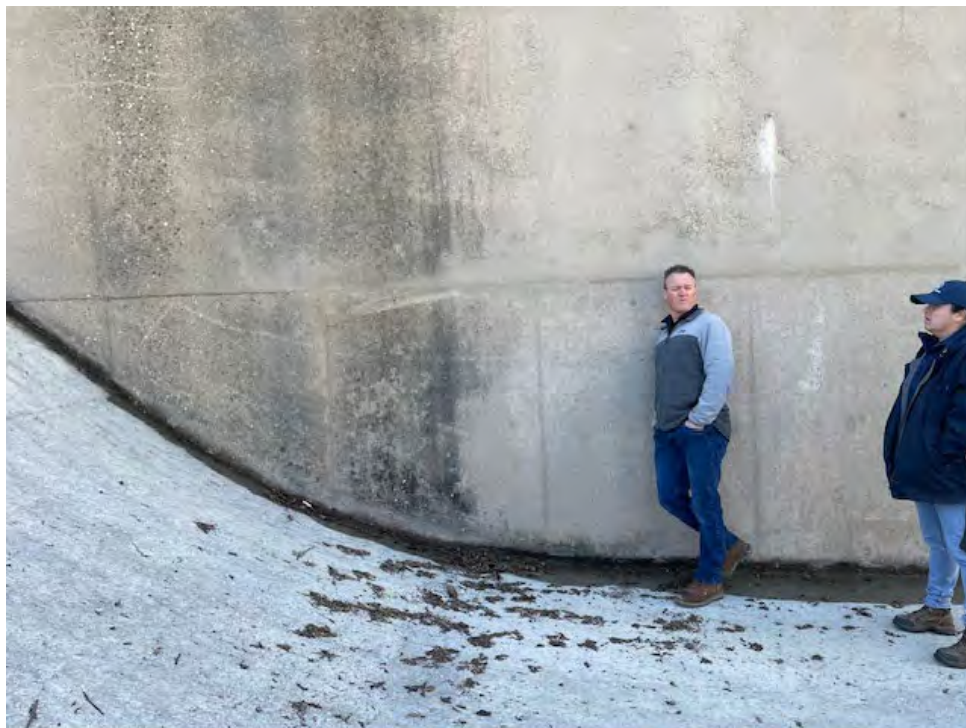
Figure 4 – Seepage at SFD Spillway on March 12, 2024
