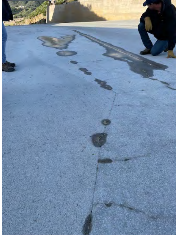
Figure 3 – Seepage at SFD Spillway on March 12, 2024
