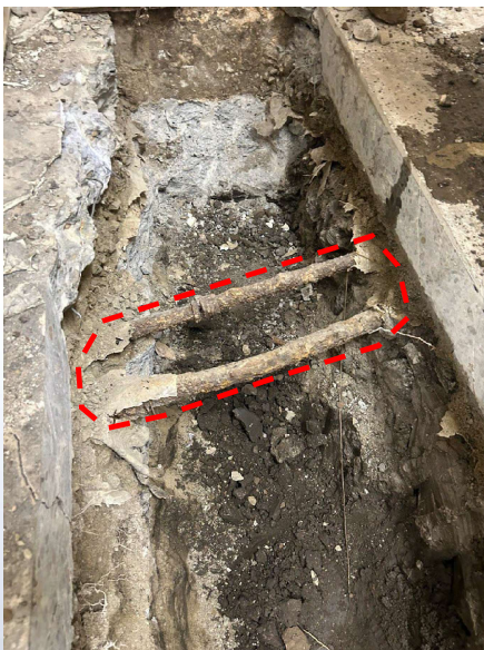
Corroded electrical conduit in slab (seven Locations)
